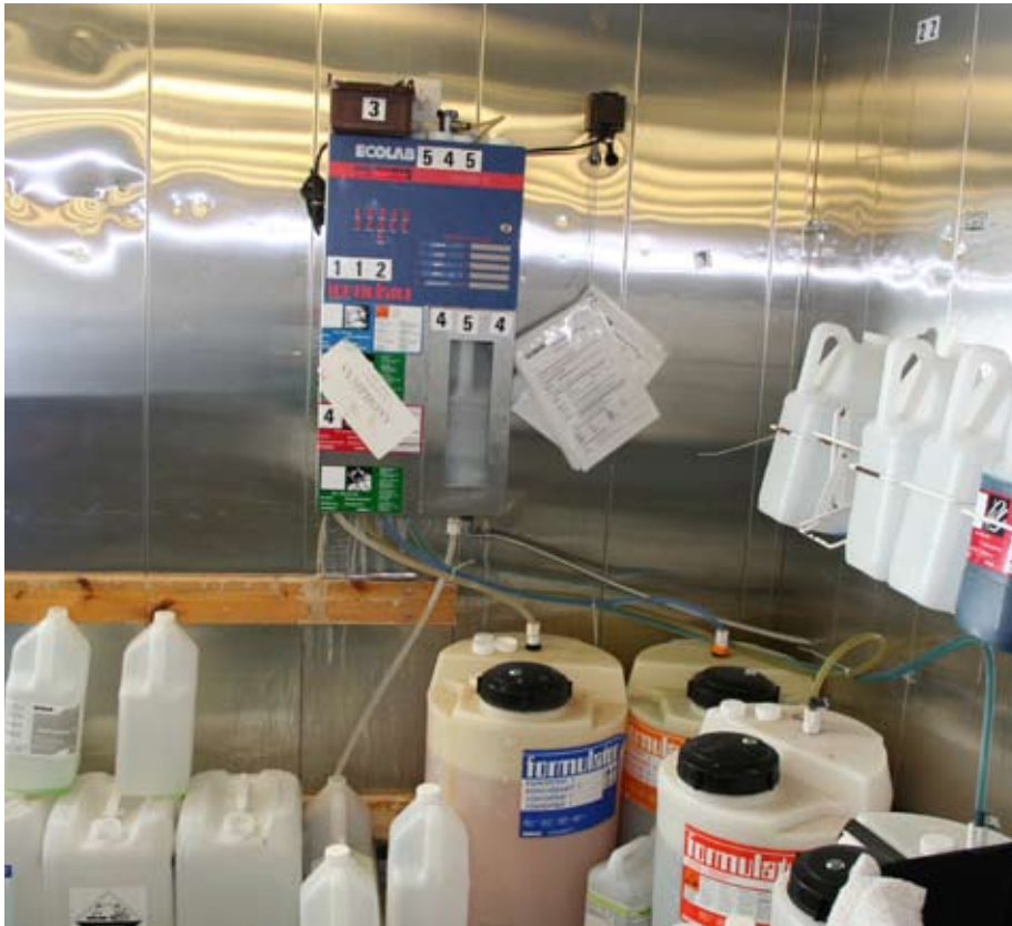
Cleaning products for the kitchen are all mixed using a dosing machine.
