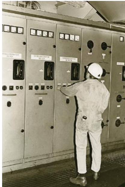
Not much has happened in planning of control rooms since this picture was taken, despite new instruments requiring different procedures and working positions.
