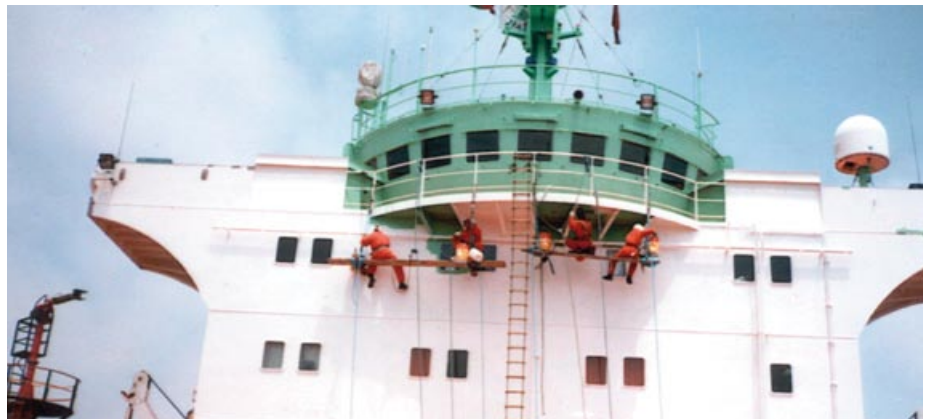
Working at great heights may be risky if crewmembers are not in balance.
