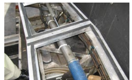
In the centre part of the photograph, the rudder posts can be seen and the damage caused to the hull lead-through.
