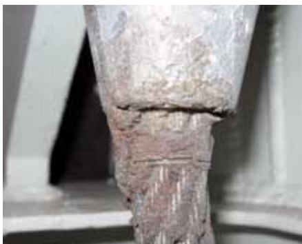
Wire has started to slip out of the spelter socket (close-up).
