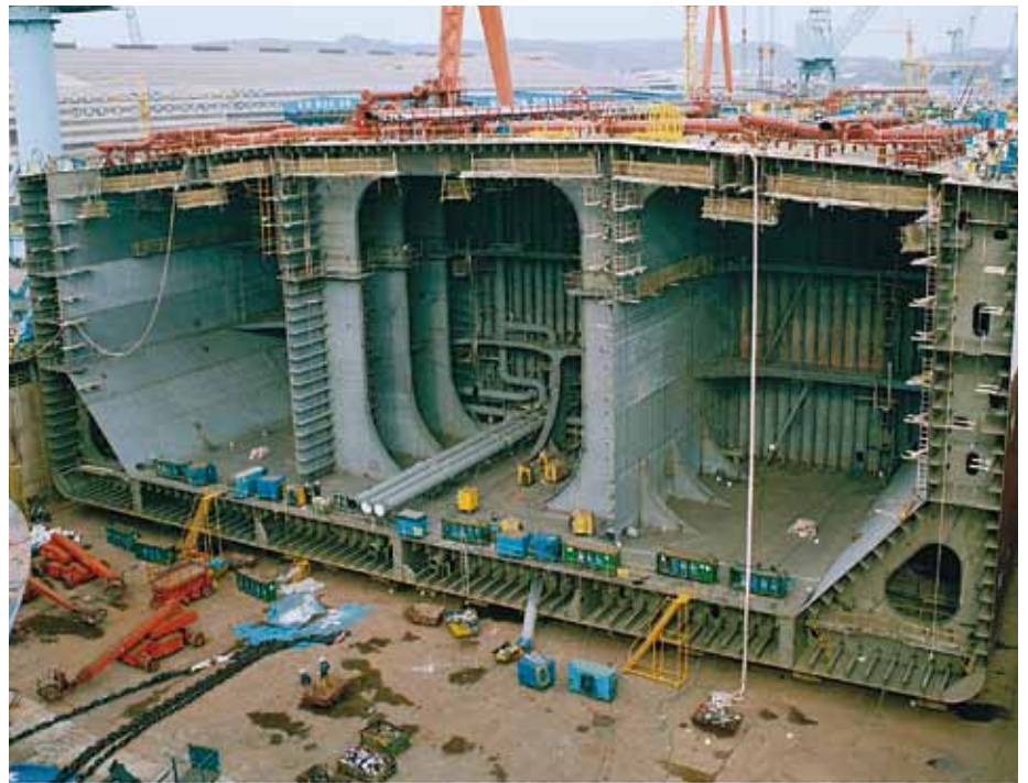
Mistakes that are built in at the shipyard are often expensive and difficult to change at a later stage. Photo Stena AB.
